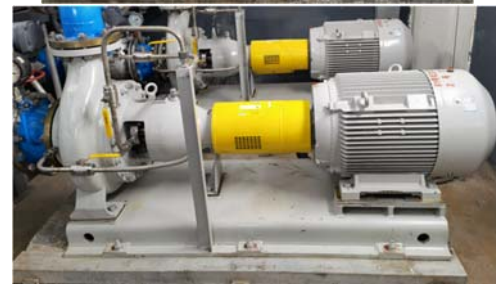
FIGURE 7: INSTALLATION EFFECT OF NEW AND OLD CENTRIFUGAL PUMPS
